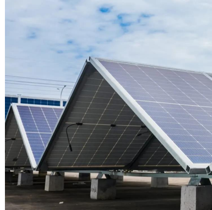
Shipping Container Solar Systems in Remote ...
