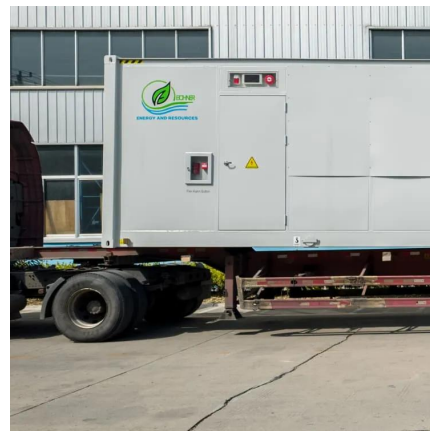
MV-inverter station: centerpiece of the PV eBoP solution
