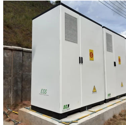
Huawei Somalia energy storage equipment
