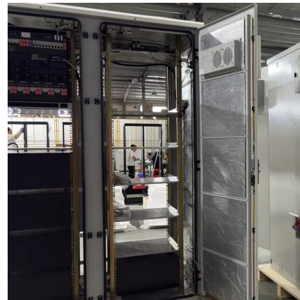
Photovoltaic Power Supply System for ...
