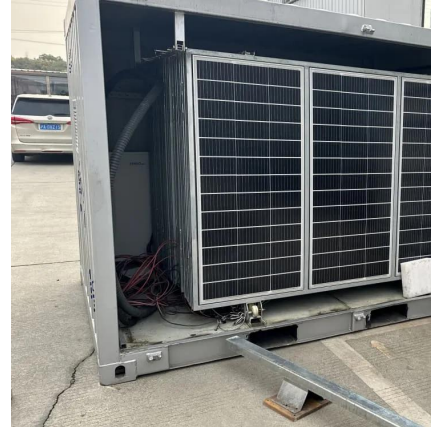
Onsite Solar , ENGIE Impact
