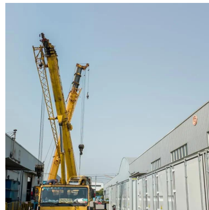
CATL's TENER Stack: 9 MWh Containerized Stacked BESS ...
