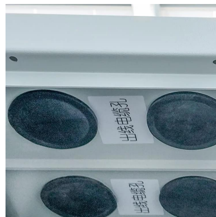
Energy storage containers: an innovative tool in the green energy ...
