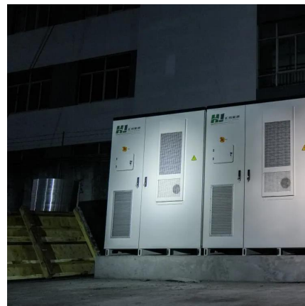
CONTAINERISED HYDROGEN FUEL CELLS ...
