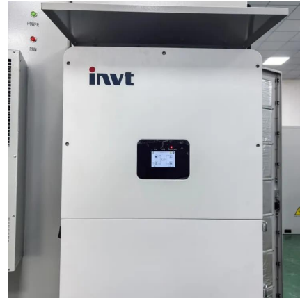
Honiara multifunctional communication base station ...
