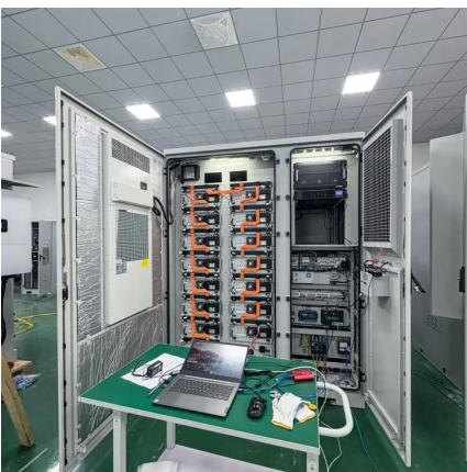
2MWh Energy Storage System With 1MW ...
