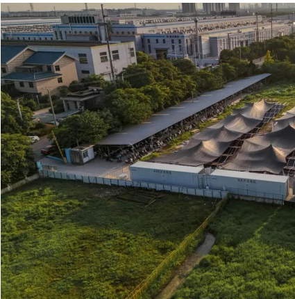
2MWh Energy Storage Container System
