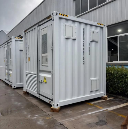
Kuwait industrial battery energy storage system
