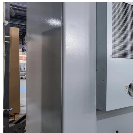
Bolivia 10kV Energy Storage Power Station
